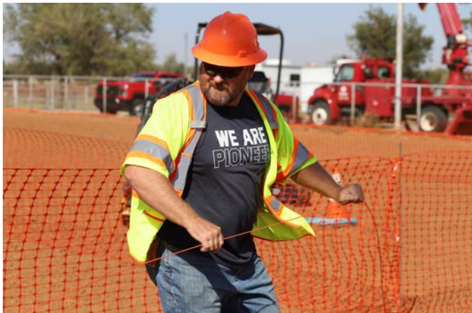
Lynn Stout, Lead Outside Operations, demonstrates fiber installation techniques during the 'Install Rodeo,' part of the employee meeting's hands-on education experience.
